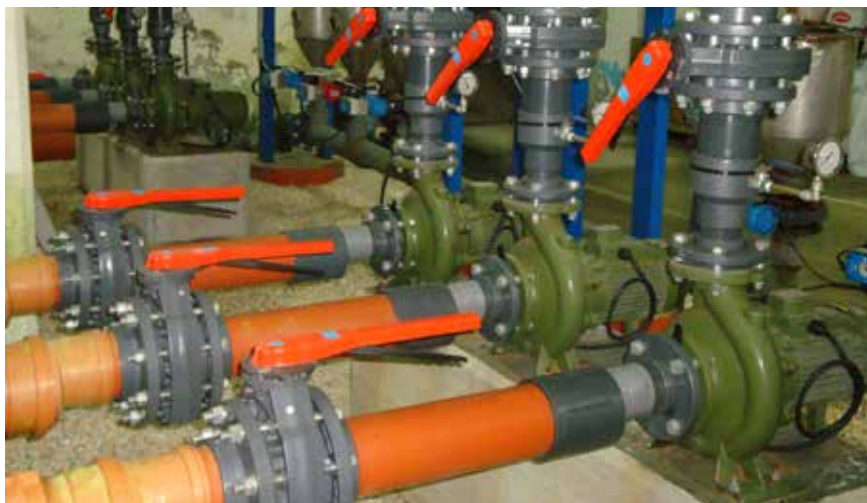
NR. 25 IR4P 65-250NB SPAIN PVC PRODUCTION PLANT
